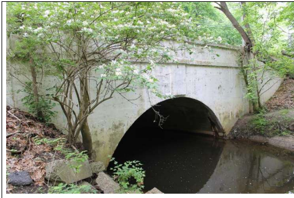
Photograph 5: North (downstream) elevation prior to the rehabilitation. Looking southwest. Note the barrel arch (May 2014).
