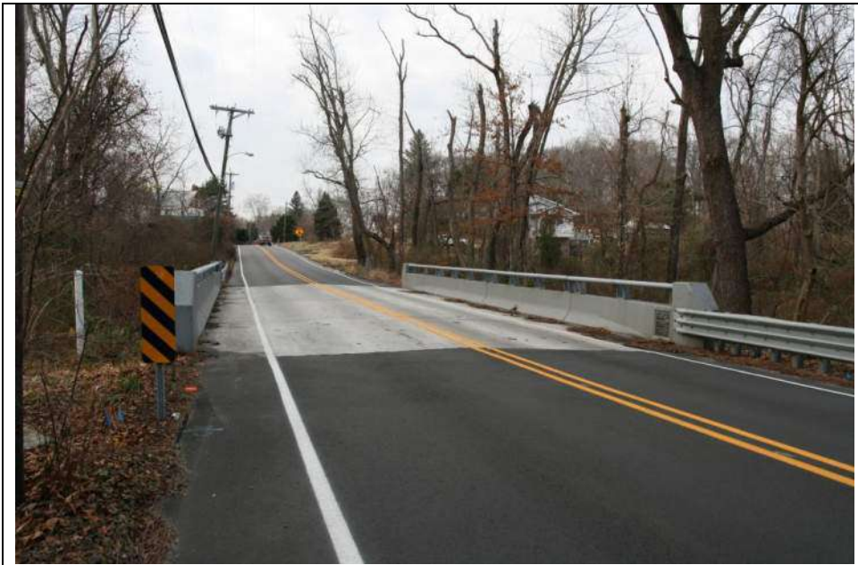
Photograph 2: Overview of the bridge, looking northwest from the east end. Note the concrete parapets with integral metal guiderails (December 2018).
