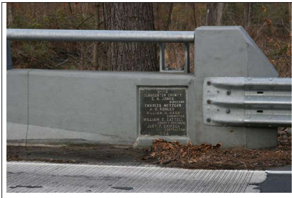
Photograph 8: Detail view of inscribed concrete bridge plaque located in the south face of the south parapet (moved from original location during rehabilitation). Looking northeast (December 2018).
