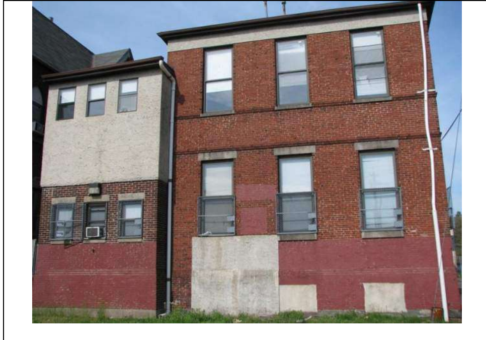
Photograph 7: East (side) elevations of the circa -1900 rear addition (right) and one of the two circa -1994 additions (left). Looking west (May 2014).
