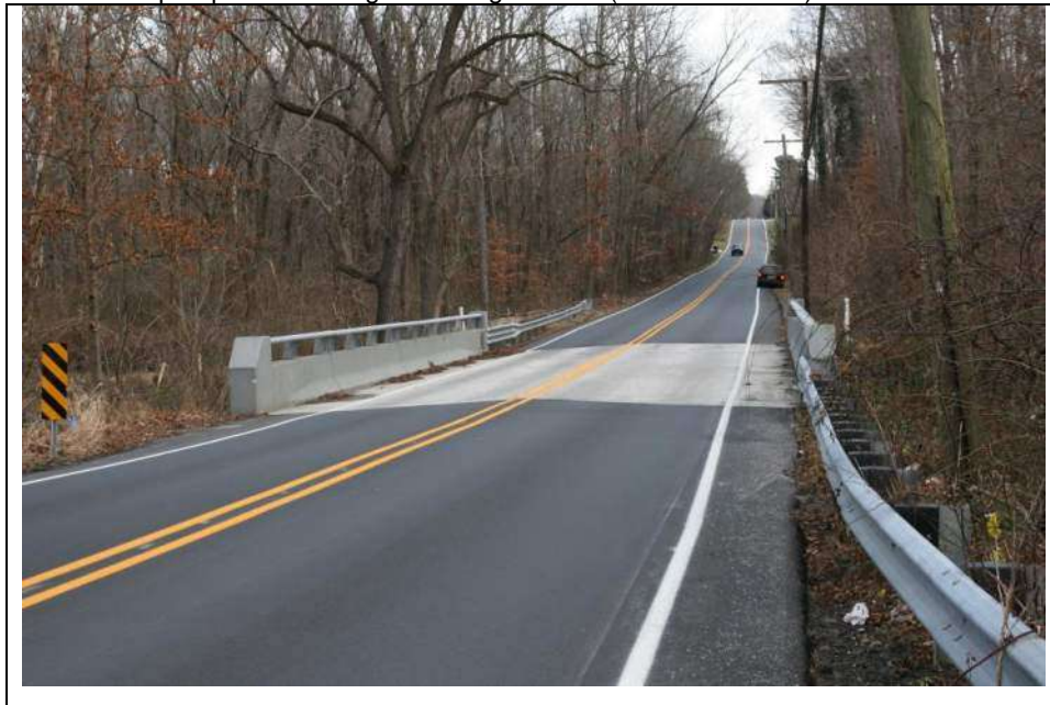
Photograph 1: Overview of the Tylers Mill Road Bridge over Chestnut Branch, looking southeast from the west end. Note the recently replaced concrete parapets with integral metal guiderails (December 2018).
